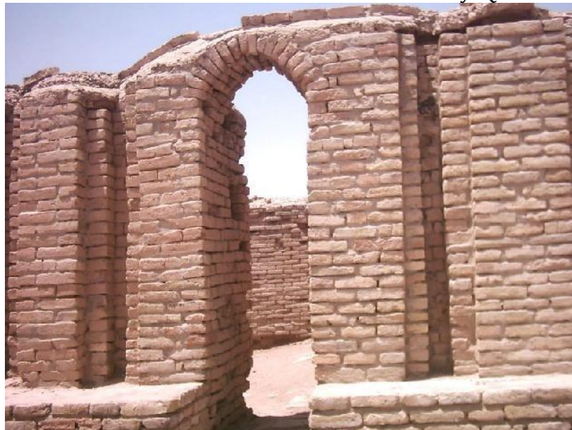
Figure 2-29: The main entrance of the E-dub-lal-mah in Ur. By: Qahtan Al Abeed, 2011
