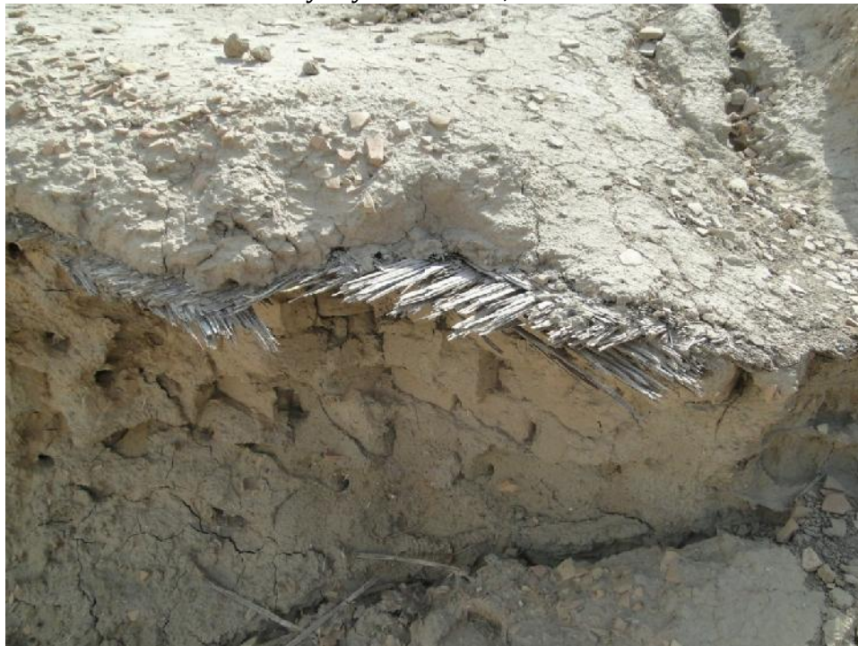
Figure 2-19: Reedmat Between Layers of Mubrick in the Inanna Ziggurat in Uruk. By: Ayad Kadhum, 2013
